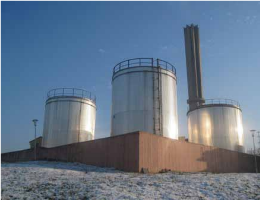
Public heating company of Prishtina - Termokos
